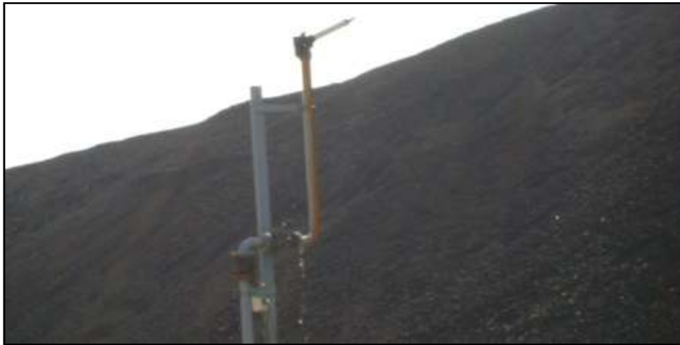
Photograph of sprinkler at coal stacker
