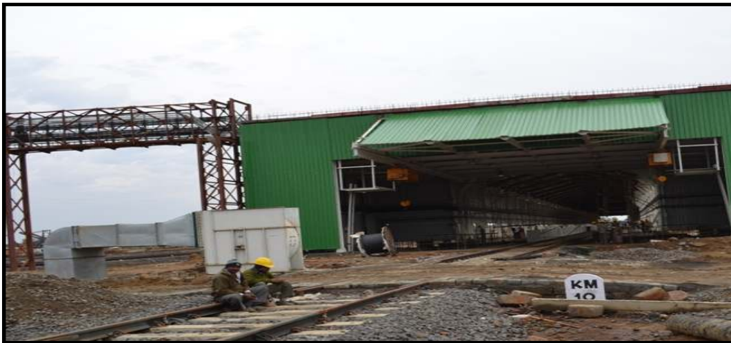
Coal wagon unloading system
