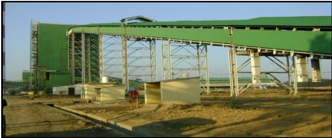
CHP and covered conveyer belts
