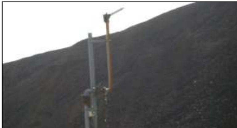
Photograph of sprinkler at coal stacker
