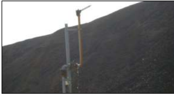
Photograph of sprinkler at coal stacker
