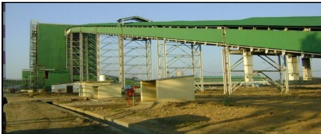
CHP and covered conveyer belts
